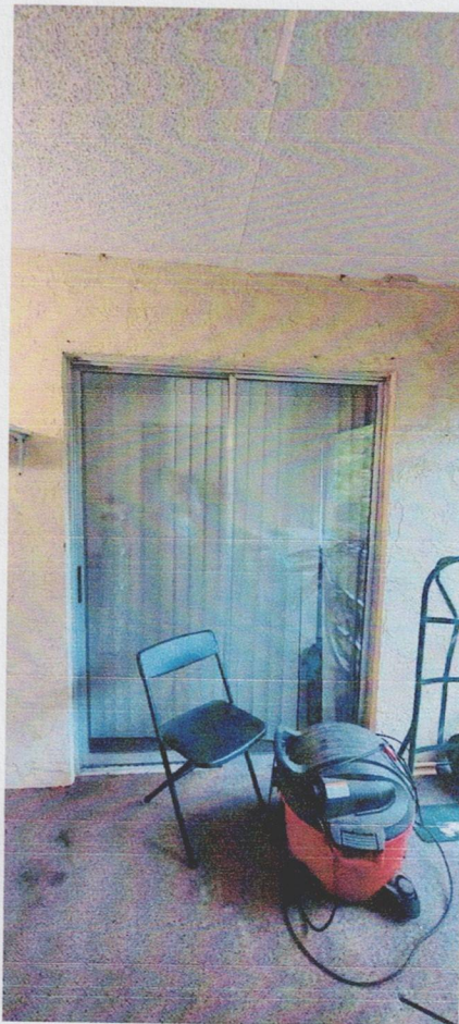
Unprotected glazed entry door
