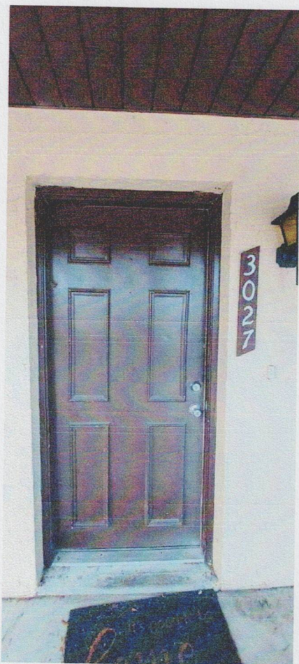
Unprotected non-glazed entry door
